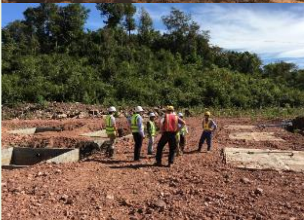
Top photo shows construction of wastewater pond replanted with aquatic plants to create a wetlands treatment pond. However, the pond is not properly lined and the selected plants do not meet wetlands plant criteria. Bottom photo shows improperly constructed treatment plant.
