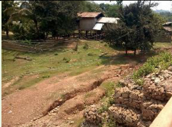
Erosion at the bridge on the Dam Access Road at Ban Thaheua , Zone 3
