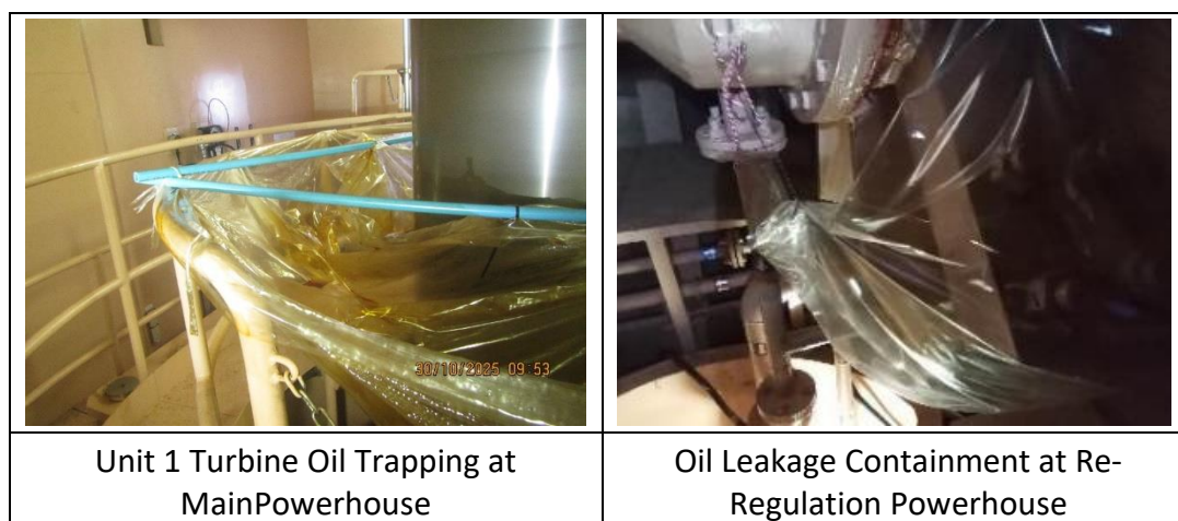
FIGURE 2.5-1: OIL LEAKAGE FROM THE UNIT 1 TURBINE WITHIN THE MAIN POWERHOUSE AND RE-REGULATION DAM POWERHOUSE
