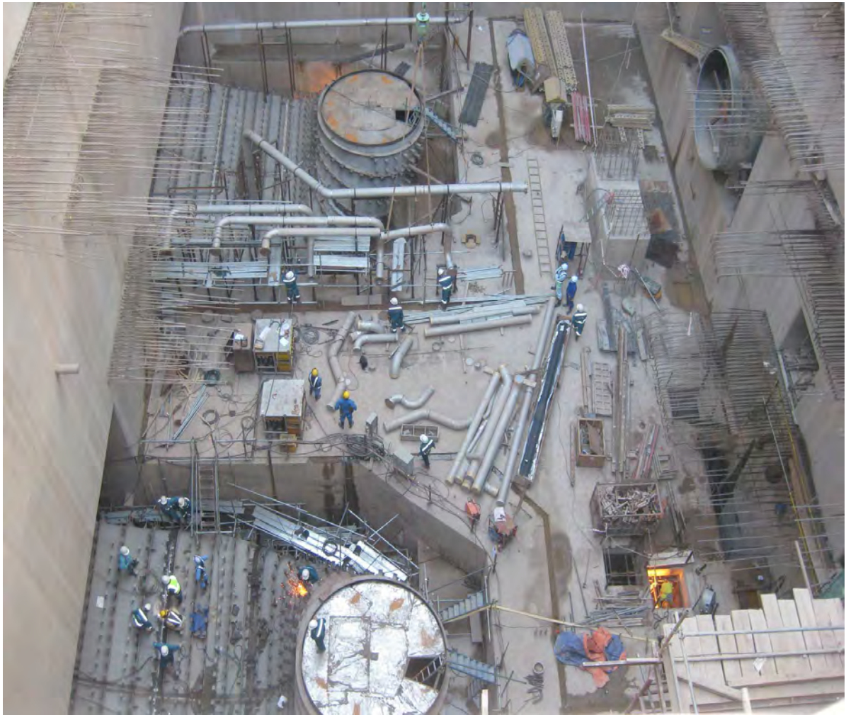
Turbine Pit Unit No. 1 & 2
